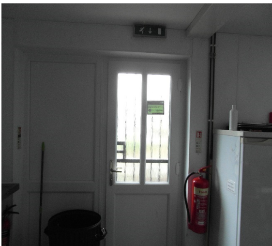
Kitchen fire exit
