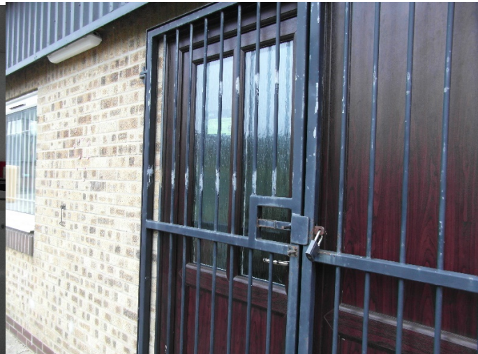
kitchen fire exit blocked with gate
